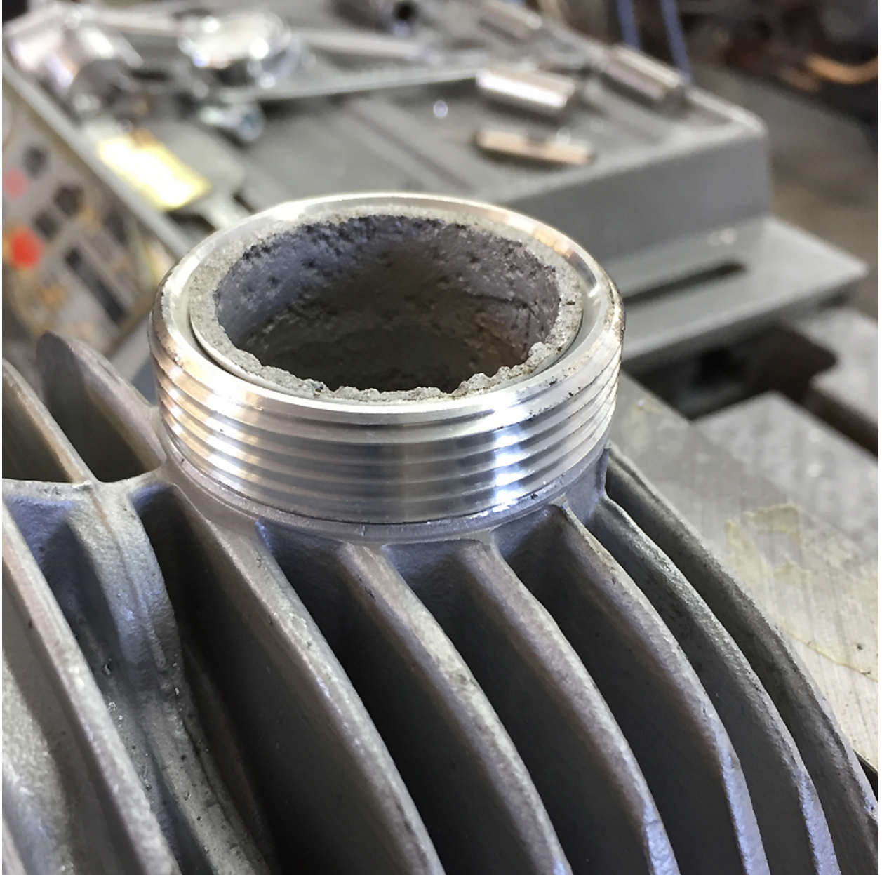
Corroded and pitted port:
